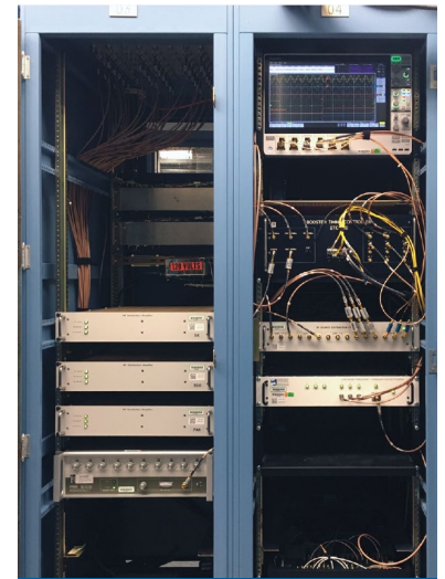
Injection/extraction timing and synchronization system (IETS)
