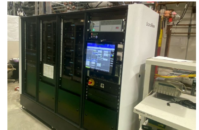
50-MW K2 klystron and modulator
