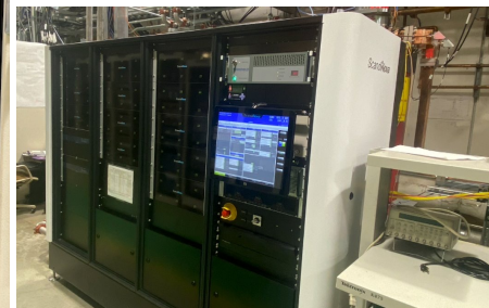
50-MW K2 klystron and modulator
