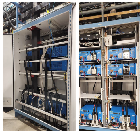
Power supply racks
