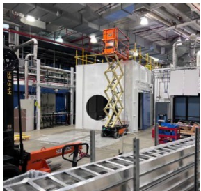
9-ID shielded enclosure
