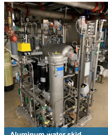
Aluminum water skid installation
