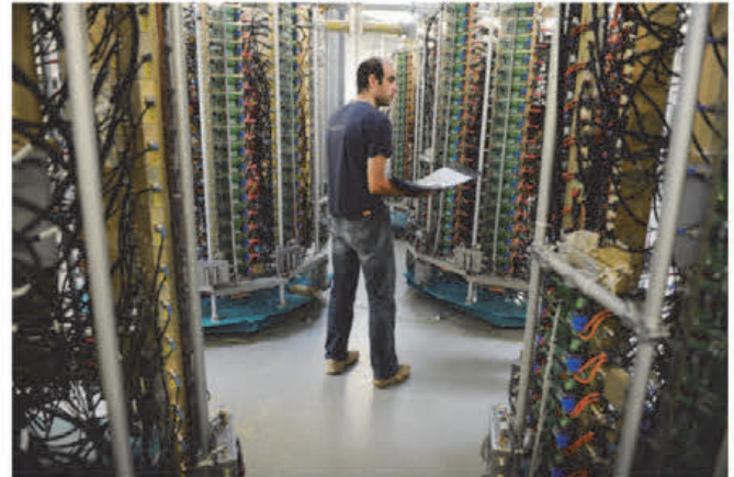
Towers of Solid state amplifiers, which power the accelerating cavities cryomodules of SOLEIL's storage ring. This technology was transferred to a French company.
