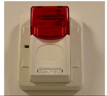
Photo of the Warning Light in the Gowning Room
