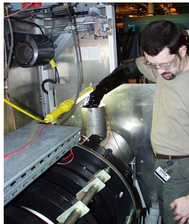
Ground-stick terminals inside tank before entering!
