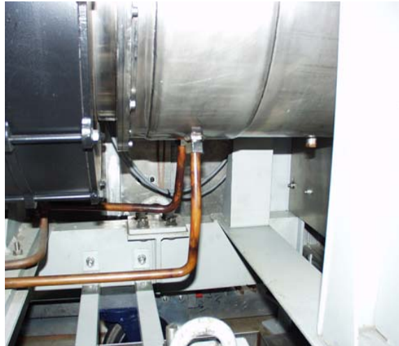
TH2089A oil tank water jacket
