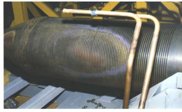
Overheated appearance on collector
