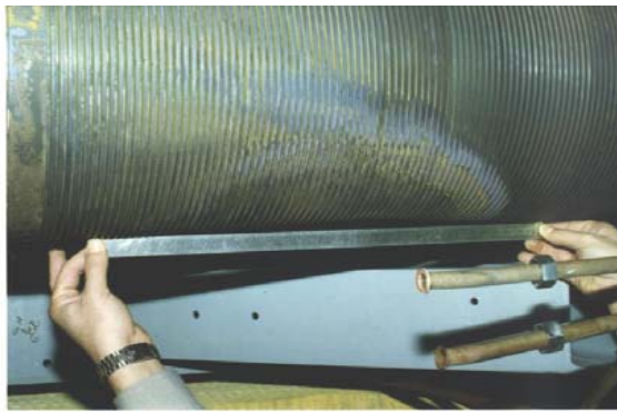
Distorted collector due to melting
