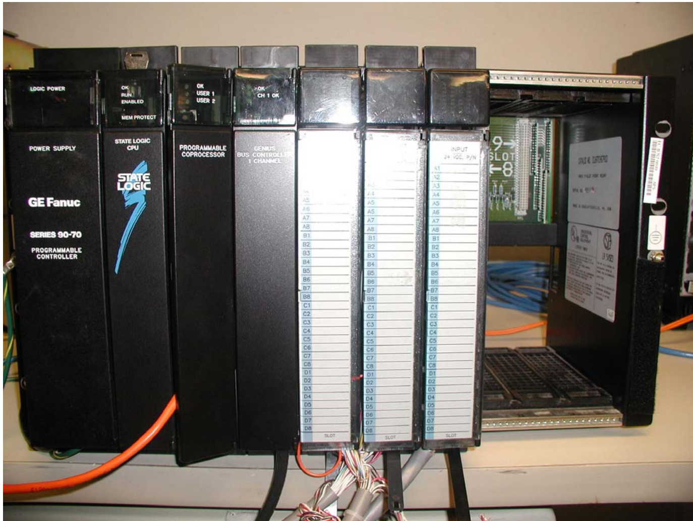
PSS Gen-1 Current Chain B Local Chassis Hardware
